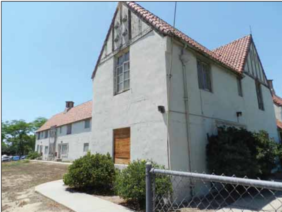
Photograph 5: Detail view showing boarded window on southeast corner of Employee Building 4; facing northwest, June 23, 2015.
