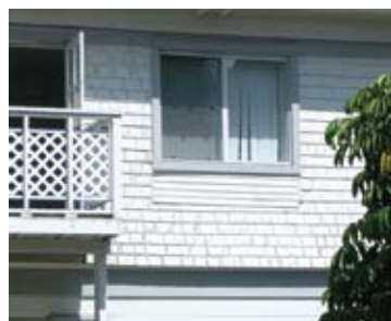
The siding added to the bottom of the window does not match the original shingle siding.
