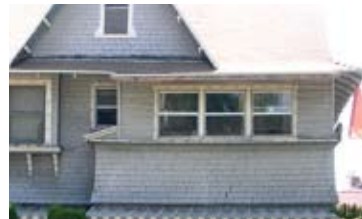
The second story balcony was altered and filled with materials that are not compatible.
