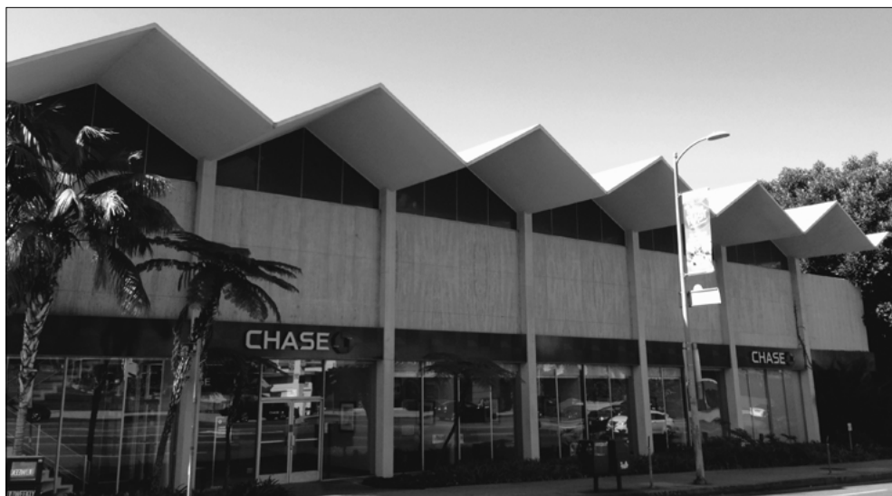
Formerly the Lytton Center, this Modern bank building with a zigzag folded-plate roof is threatened with redevelopment. Photo by Adrian Scott Fine/L.A. Conservancy.
