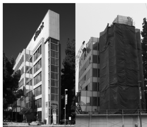
Commonwealth Savings Building before and during demolition. Photos by (l-r) John Eng and Jessica Hodgdon/L.A. Conservancy.
