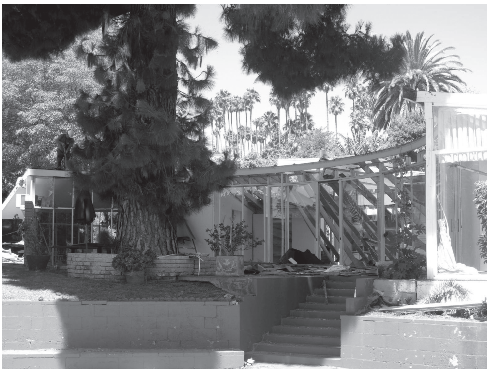
The Shusett residence (1951), designed by master architect John Lautner, during demolition. Photo courtesy Mark Haddawy.
