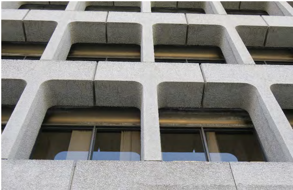
Close-up of upper floors and granite aggregate cladding at the north façade, view south (ARG, 2017).
