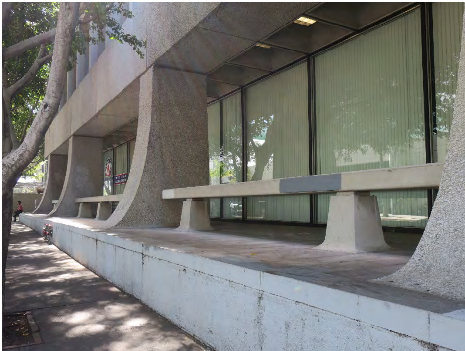
First floor exterior corridor and concrete railing at the east façade, view southwest (ARG, 2017).
