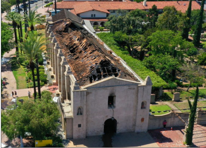
Aerial view of the fire damage sustained at Mission San Gabriel. Photo: Carolyn Cole / Los Angeles Times
