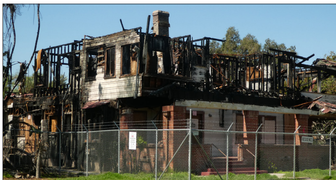
Due to neglect, buildings have been destroyed from vandalism and arson fires. Photo by Adrian Scott Fine/L.A. Conservancy
