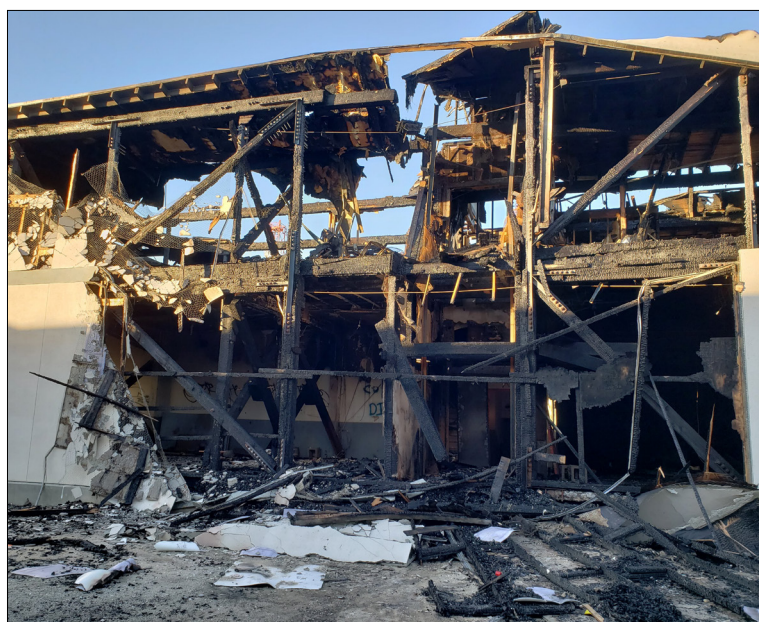
The Pickle Works building was declared a total loss after a fire broke out in 2018. Photo by Jessica Hodgdon/L.A. Conservancy.
