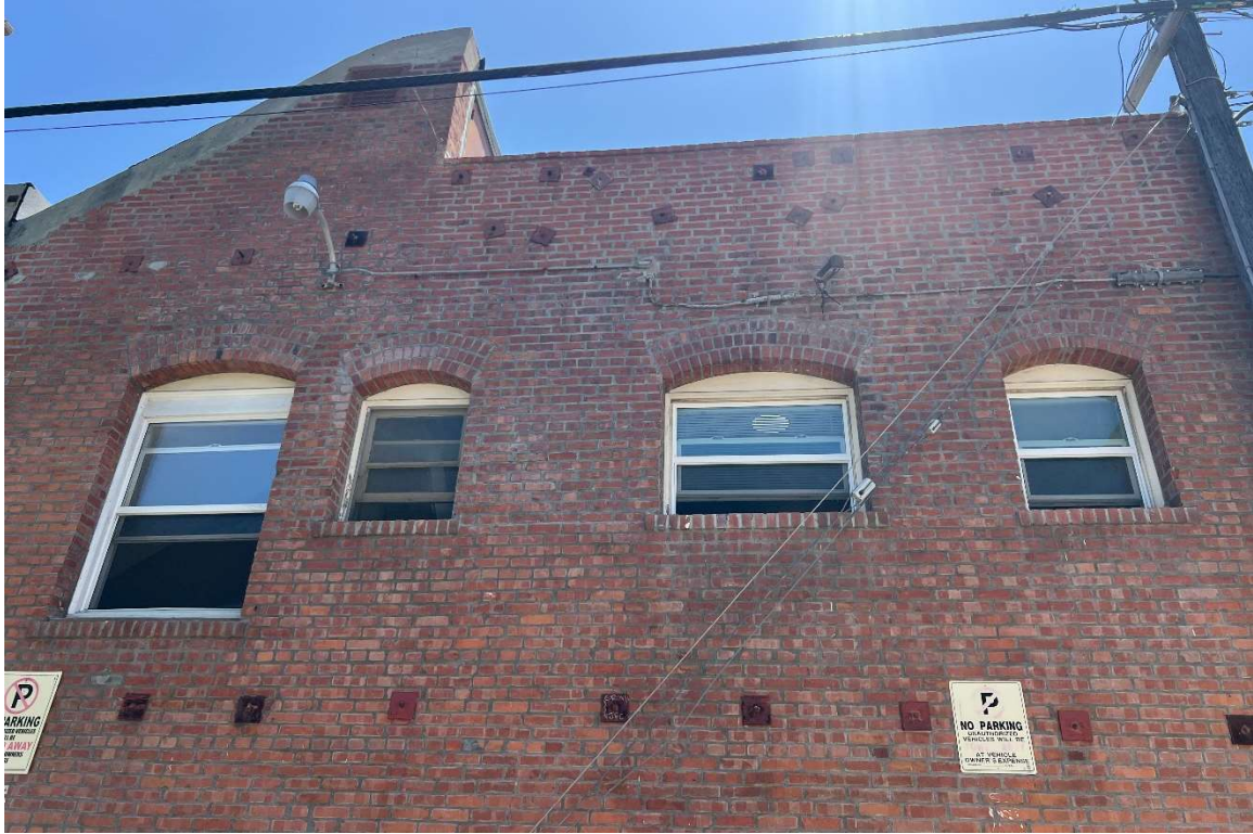
Photo 9: North façade, detail of replaced second floor windows, view south from alley
